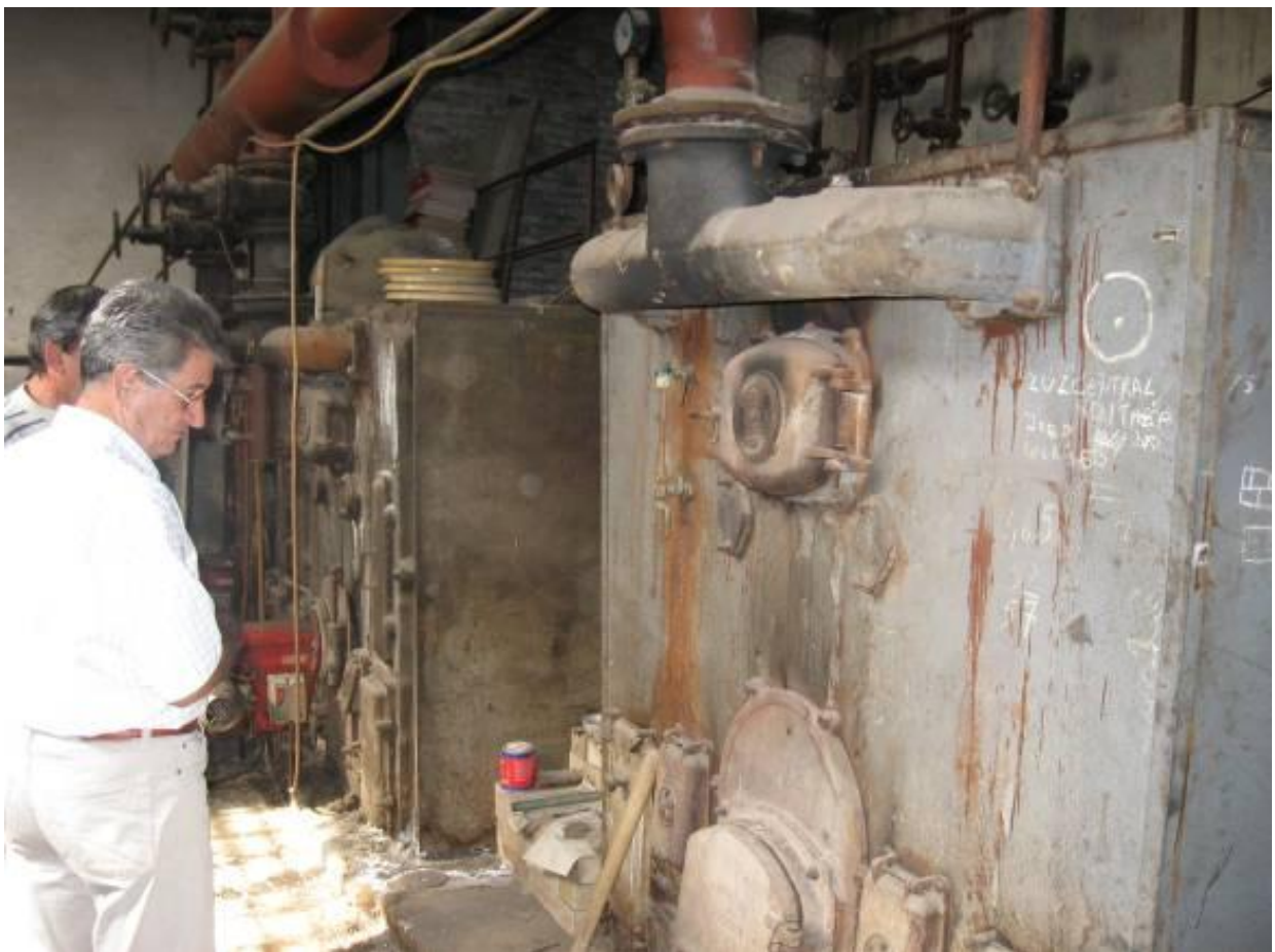
Figure 5. The wood-fired boiler from year 1959 which has not been in operation the last 15 year. This boiler needs to be demounted to make place for the new bio boiler. In the rear end are the two oil fired boilers today supplying the school with heat
